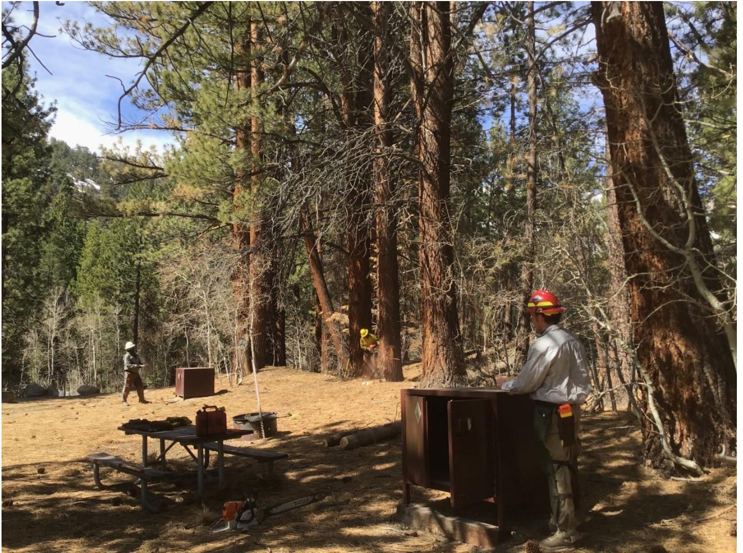
Crews falling hazard trees in Lower Lee Vining Campground (photo courtesy Mark Fogg, Bureau of Land Management)
